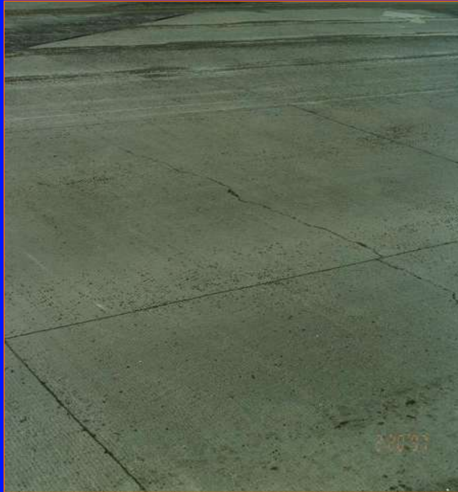
Shrinkage cracks on brand new slabs
