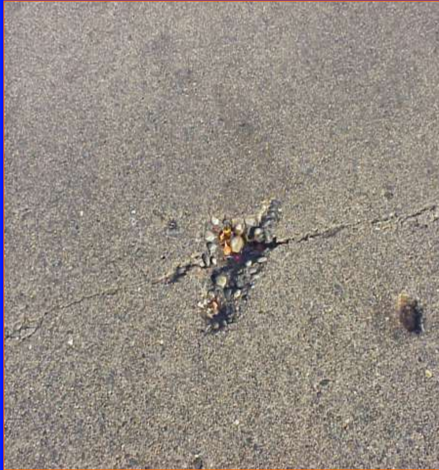
Spalling on set
