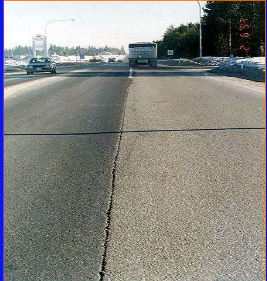
Longitudinal cracking from the poor joint construction
