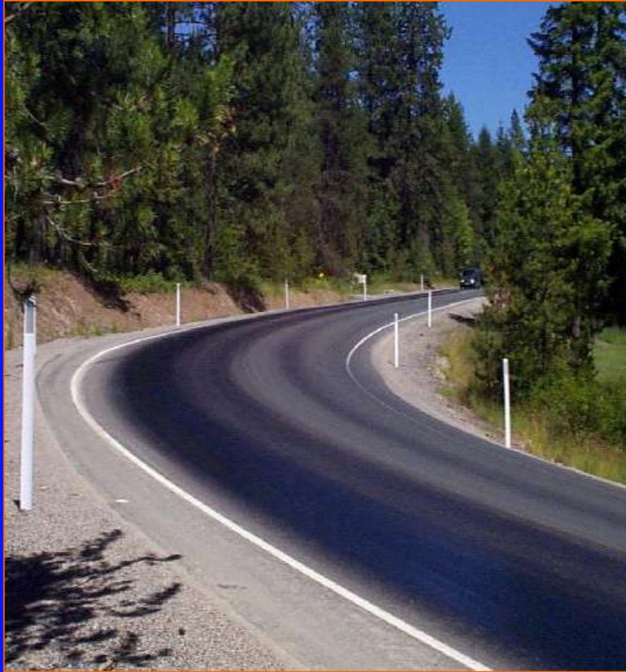
HMA bleeding on wheelpaths
