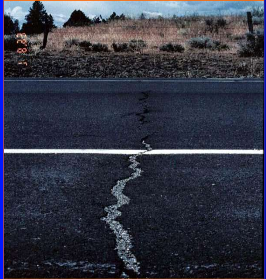
Smaller patched thermal crack
