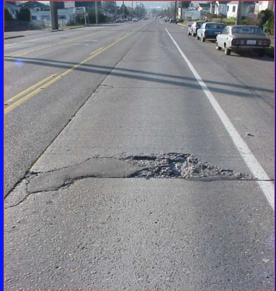
Spalling from a bad construction joint
