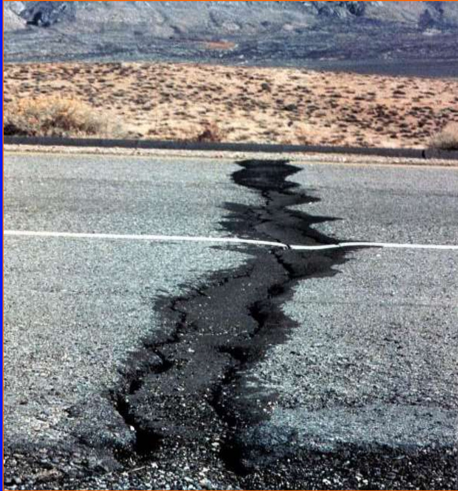
Large patched thermal crack
