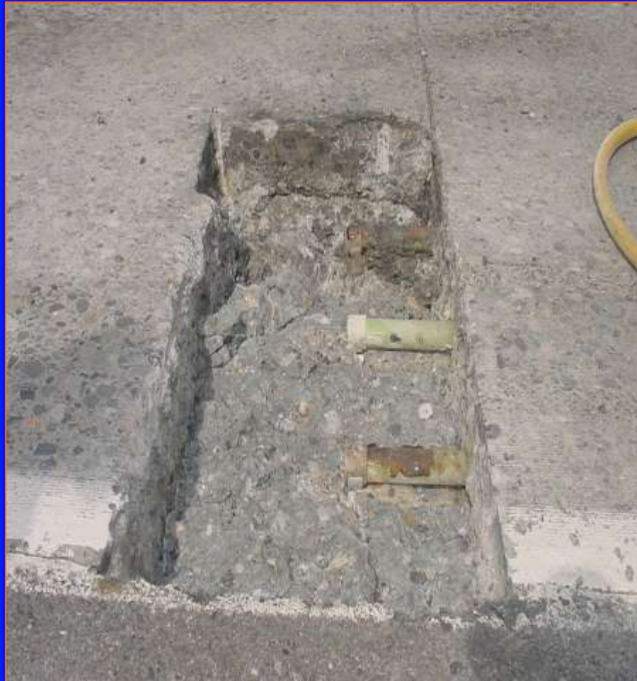
Exposed failure with rusted dowel bars
